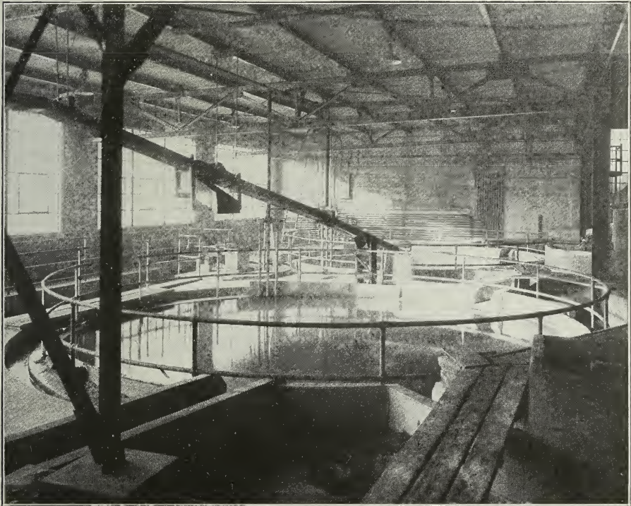
Fig. 33. Circular washers in plant of National Silica Company. Note the flume discharging into the second washer. (Photograph by courtesy of National Silica Company.)
